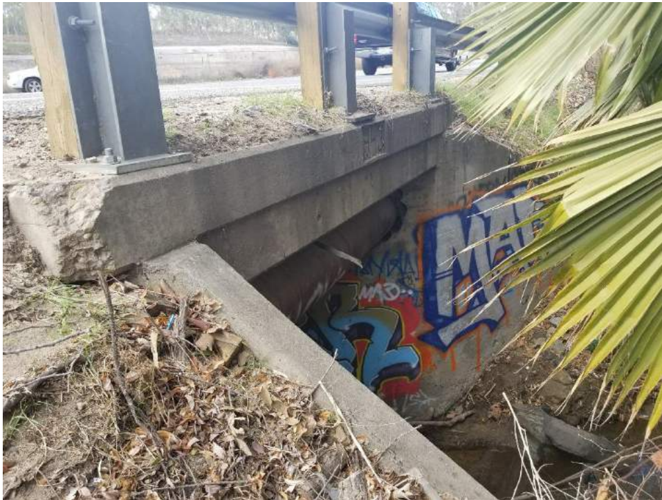
Photo 23. Collector point 395-s-011. 1943 culvert. Did not take GPS line due to traffic. Photo facing northwest. Associated with 1928 route.
