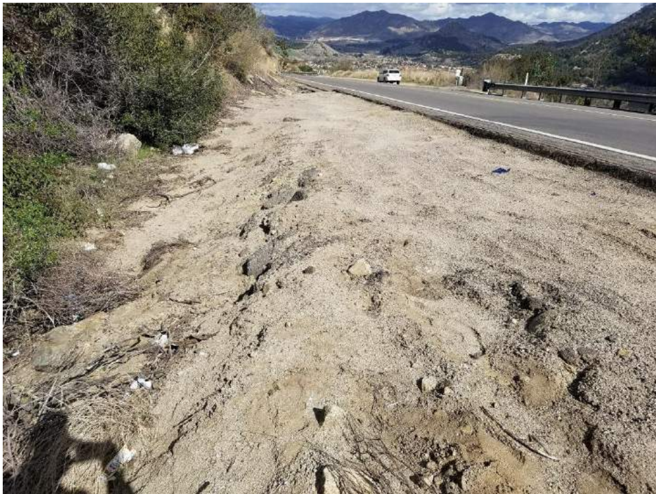
Figure 4.14.19 Small edge of road surface eroding out of soil. Facing north.
