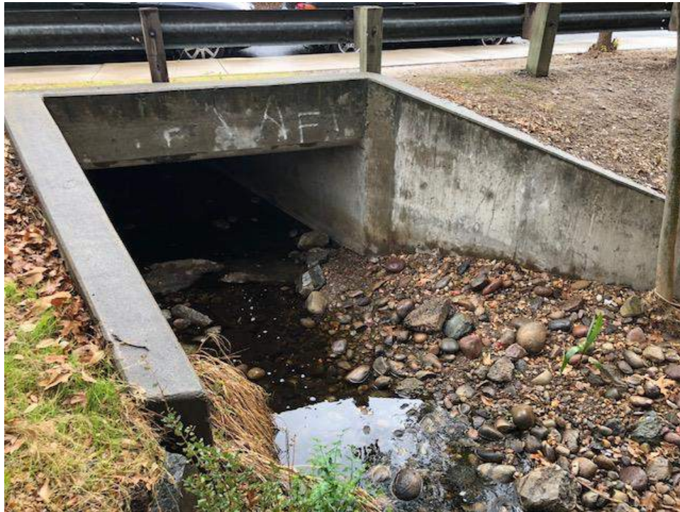
Photo 9. Possible historic culvert. On Old Pomerado Rd. Associated with 1928 route. In collector as 395-s-004. Photo facing SE.
