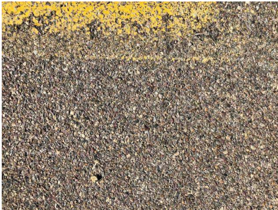
Photo 6. Historic 395 section. Abandoned. Line points in collector as 395-s-002. Close up of road material. Associated with 1928 route near Pomerado Rd.
