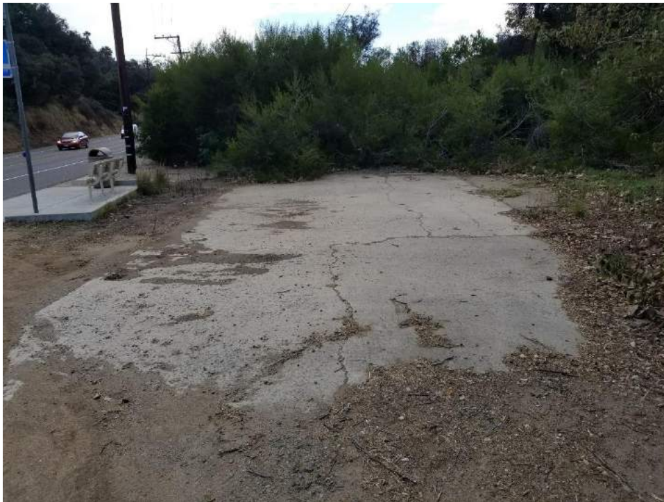
Photo 24. Collector line 395-s-012. Road section running along edge of current ROW. Photo facing south. Concrete is 18'9" wide. Asphalt shoulders are variable but at widest 5'10". Associated with 1928 route.
