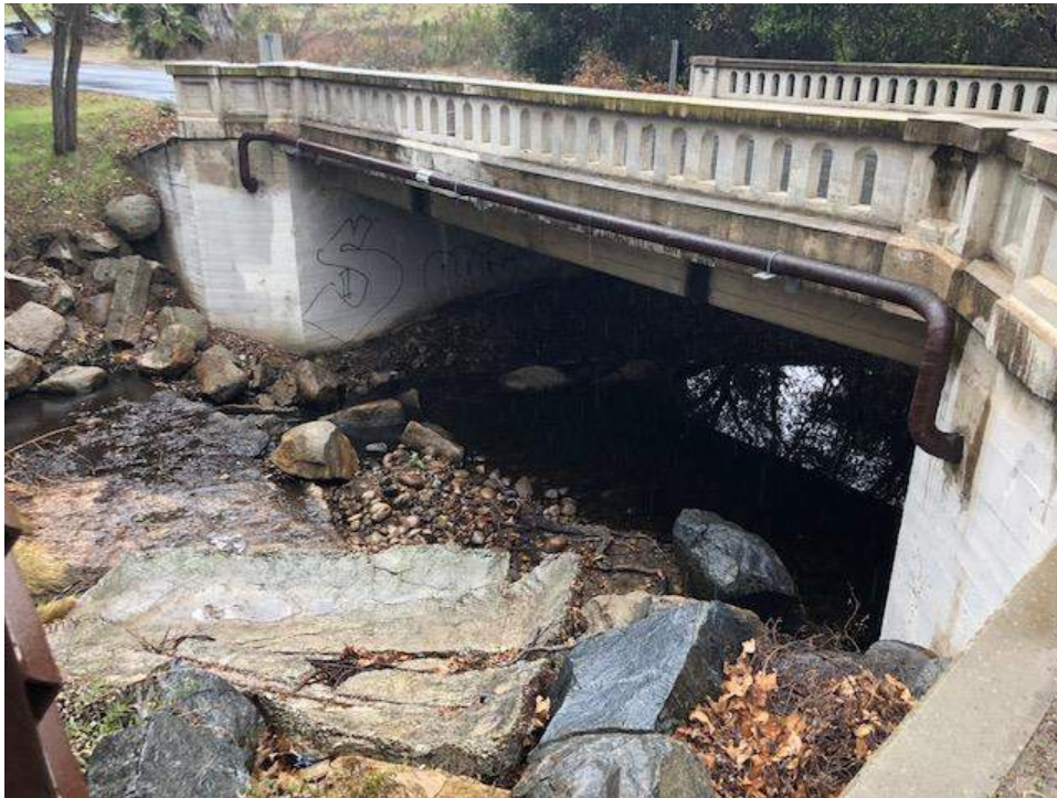
Photo 7. Historic 395 bridge. Historic bridge. Associated with 1928 route. In collector as 395-s-003. Facing West. 23.9 ft wide. On Old Pomerado Rd.
