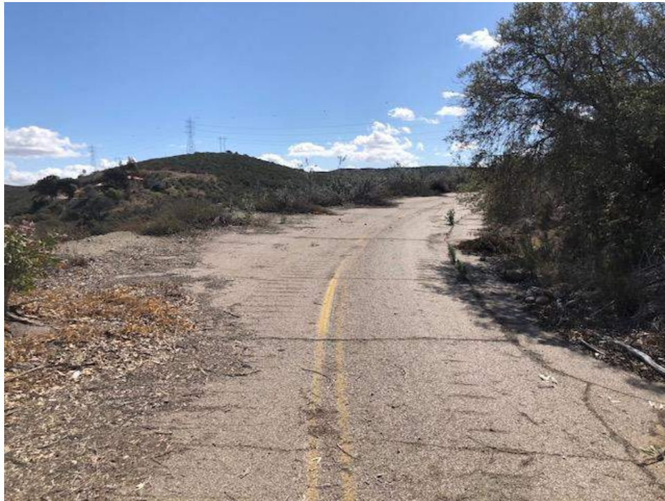
Photo 5. Historic 395 section. Abandoned. Line points in collector as 395-s-002. Facing WSW. Associated with 1928 route near Pomerado Rd. Road width 21.25 ft. Shoulder overgrown with vegetation.
