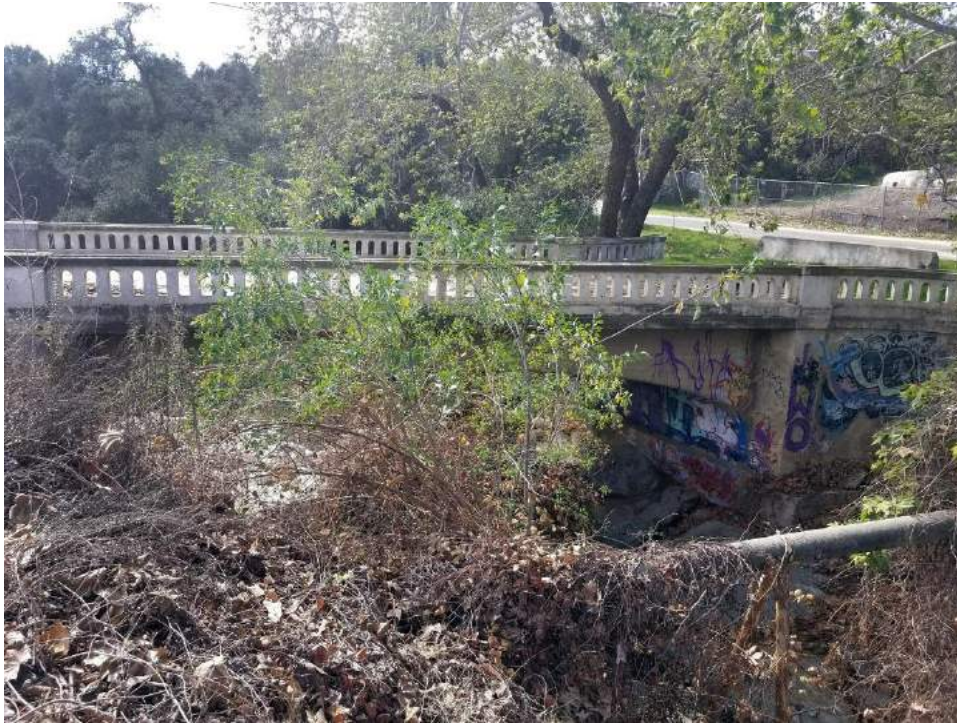
Figure 4.14.12 Bridge, facing west. Date unknown, but materials, design and style indicate 1920s.
