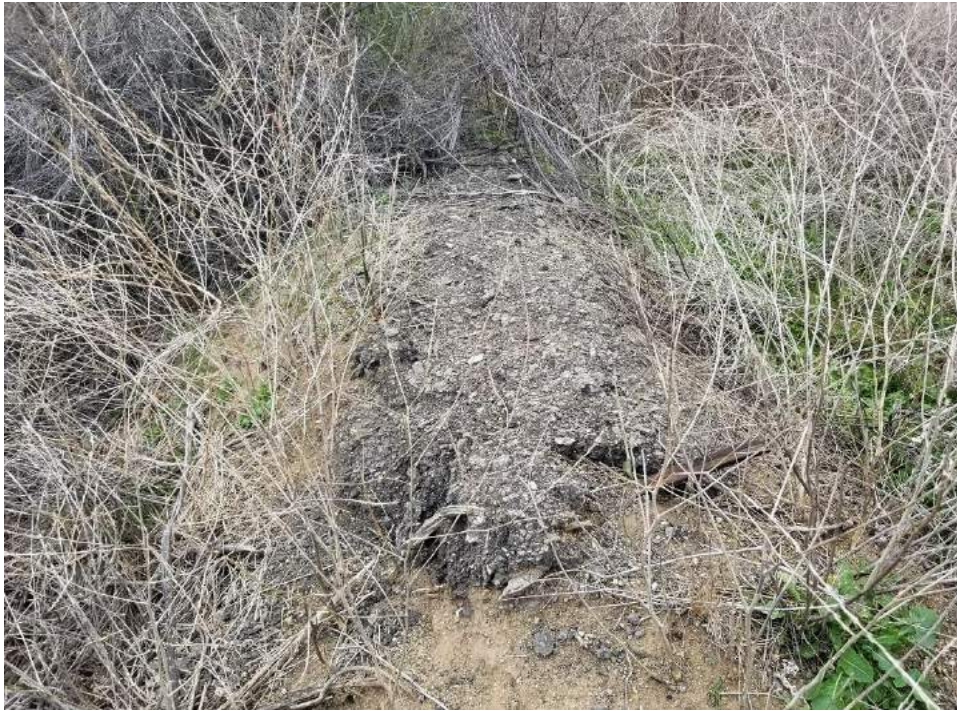
Figure 4.14.18 Small edge of road surface eroding out of soil. Facing north.
