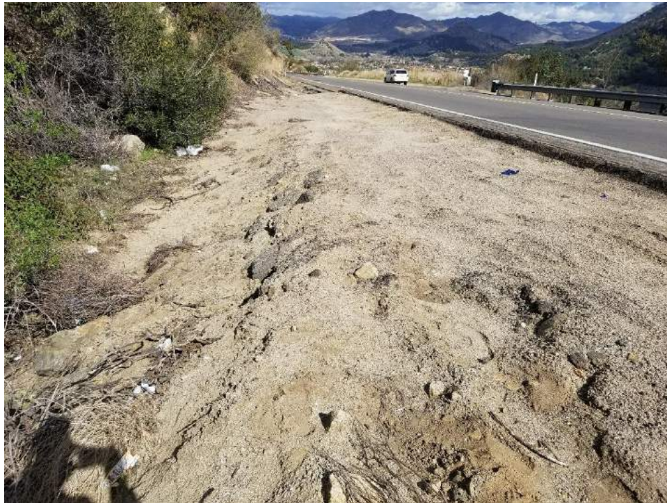
Photo 17. Collector line 395-s-008. Small edge of road surface eroding out of soil; not measurable. Photo facing north. Associated with 1948-1953 section.
