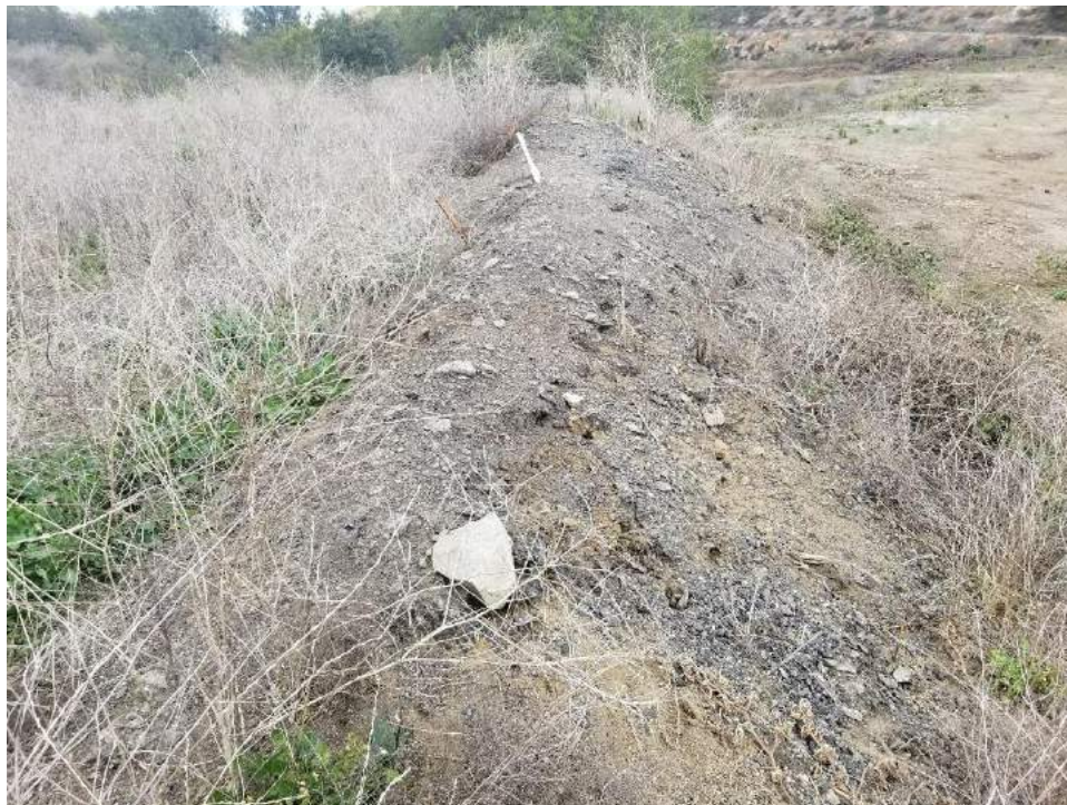
Photo 15. Collector line 395-s-007. Berm of soil and asphalt rubble bisecting 395-s-007. Facing east.
